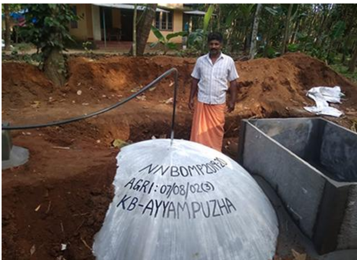
UID Number on each digester
